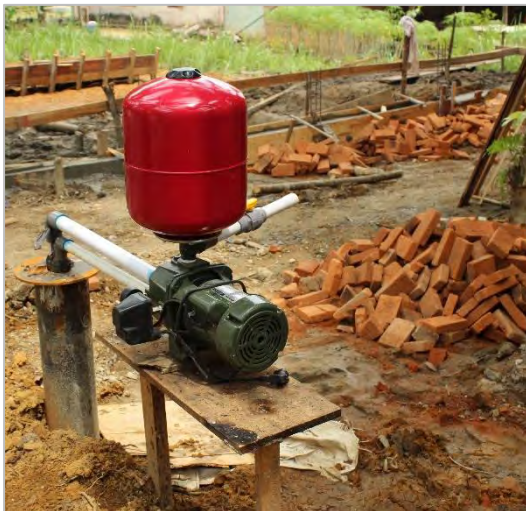
Figure 27 – Newly-built water pump in Mekar Jaya to cover water shortages. Photo taken by the author (2017).
